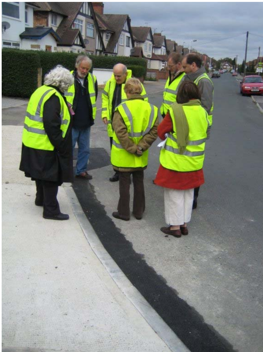
Councillors examine an 'Enviro' Kerb, made from lightweight recycled plastic, on Weald Road, Hillingdon.
