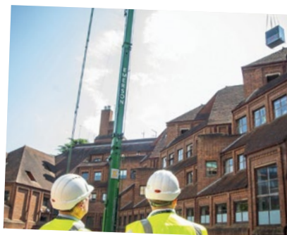
One of the largest government grants in London for our buildings' decarbonisation project
